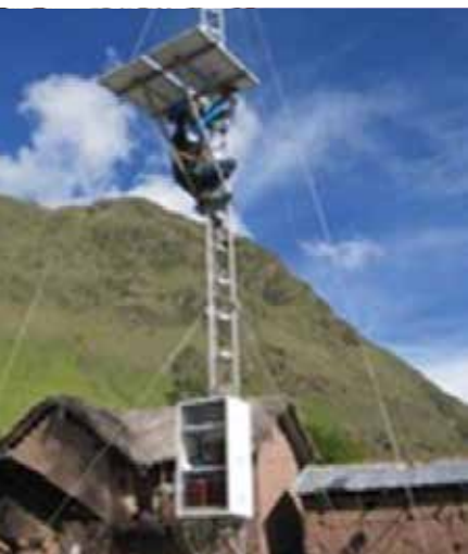
Peru – VSAT telecom tower
