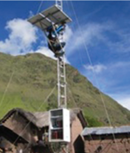
Peru – VSAT telecom tower
