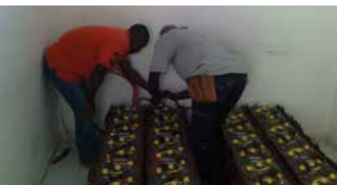
48 Trojan L16RE-2V batteries Photo by Jeff Korcan, courtesy of Solar Electric Light Fund
